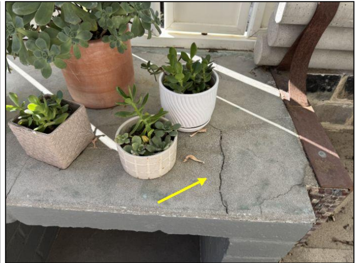
cracking on exterior concrete
