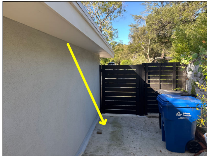
Signs of moisture falling from lack of gutters
