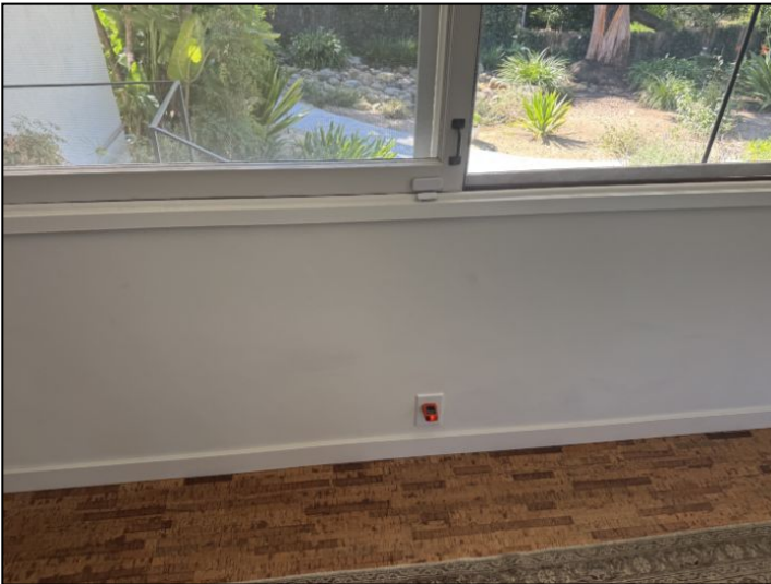
open grounds in all bedroom outlets
