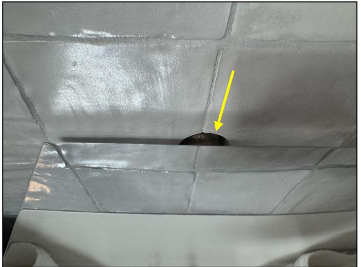
recommend sealing gap
