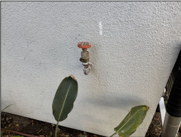
no anti siphon
