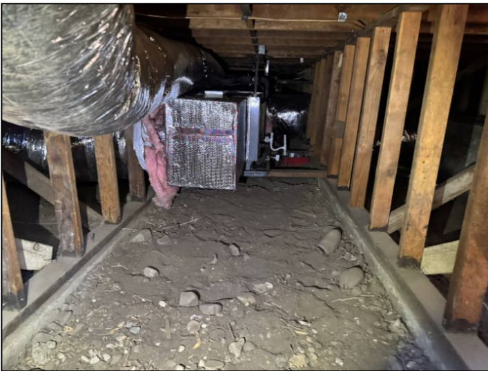
air handler location
