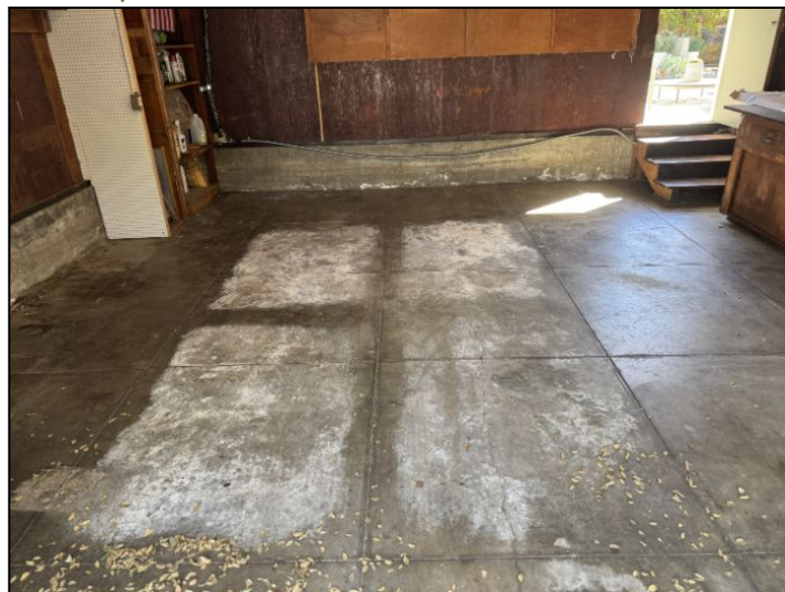
signs of moisture intrusion/mild cracking
