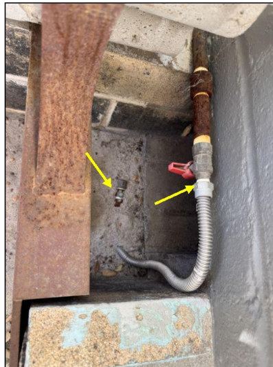
white tape on exterior gas line
