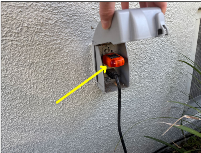
Missing gfci front of house
