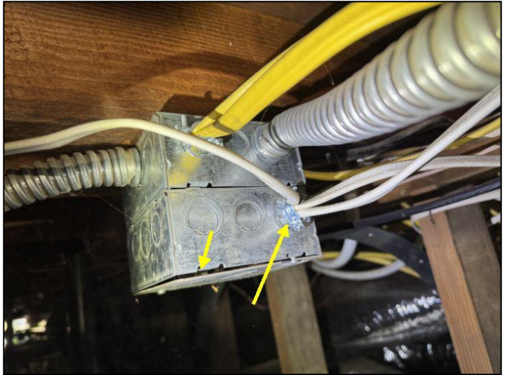
three into one/loose connection
