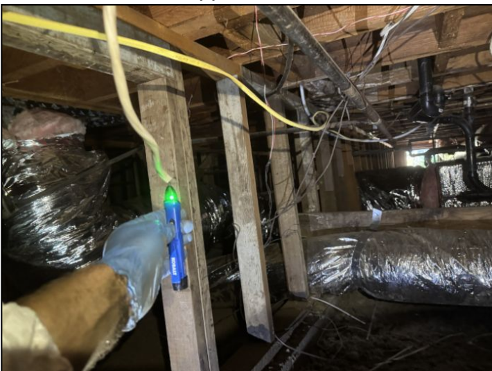
abandoned electrical- recommend removal
