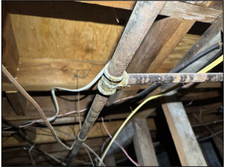
rust on gas line
