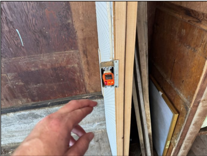
missing GFCi and cover
