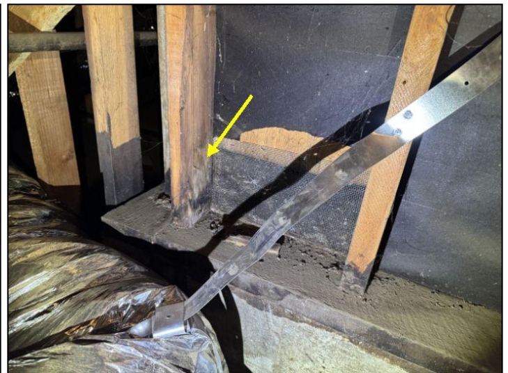
moisture at vent
