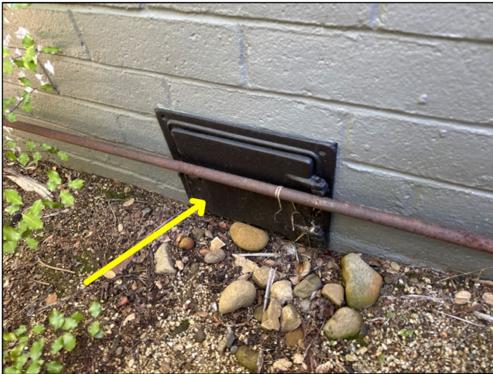
Clean out blocked
