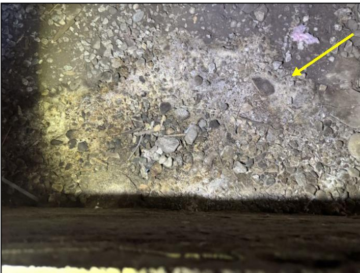
moisture at crawlspace entrance
