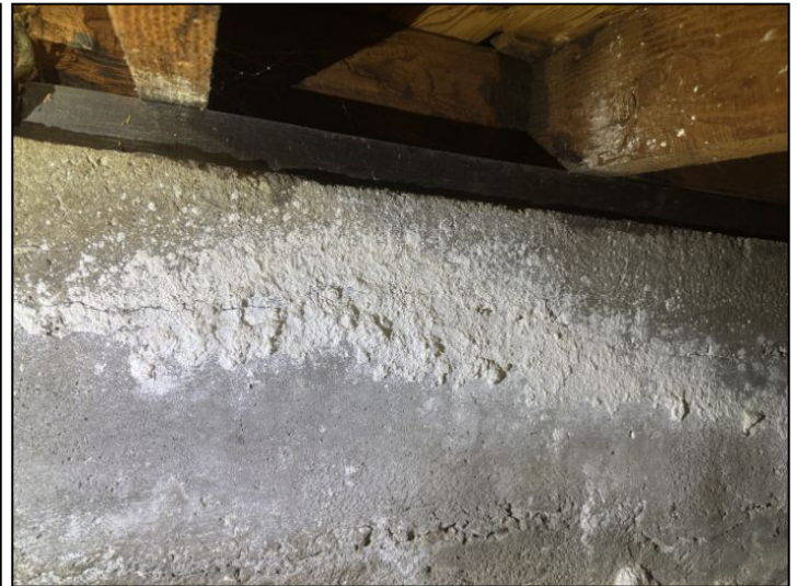
horizontal crack with signs of moisture
