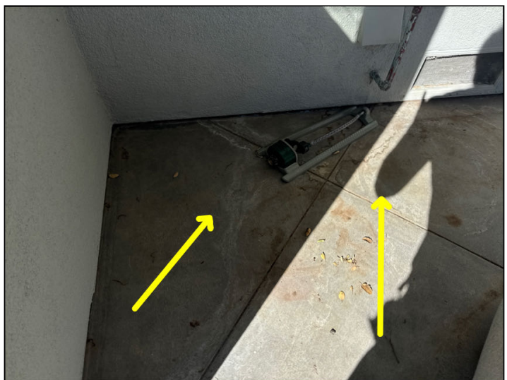
signs of moisture settlement
