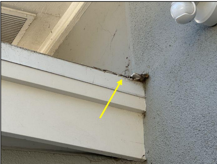
seal cracks/gaps- above garage
