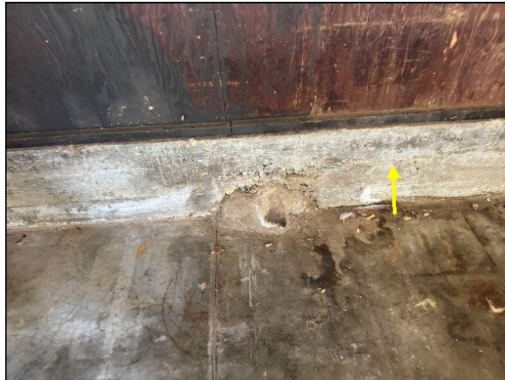
seal cracking from rock
