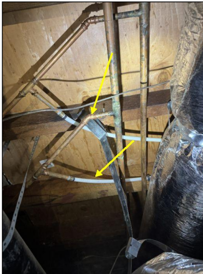
plastic piping patch
