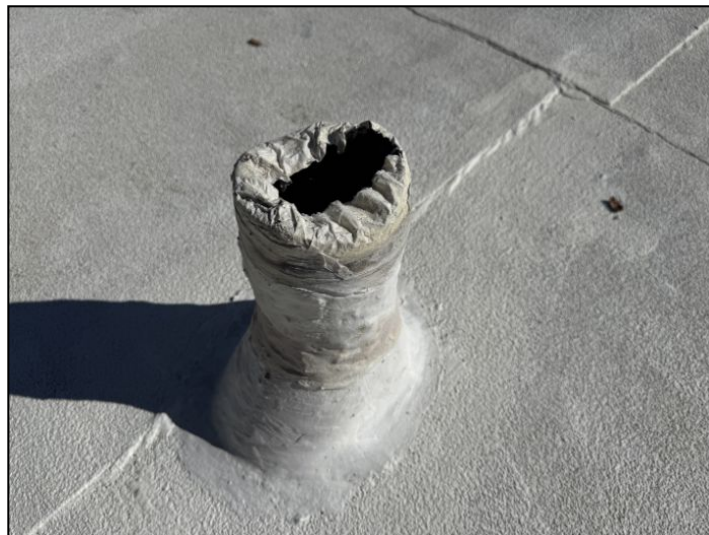
roof plumbing stack - possible asbestos
