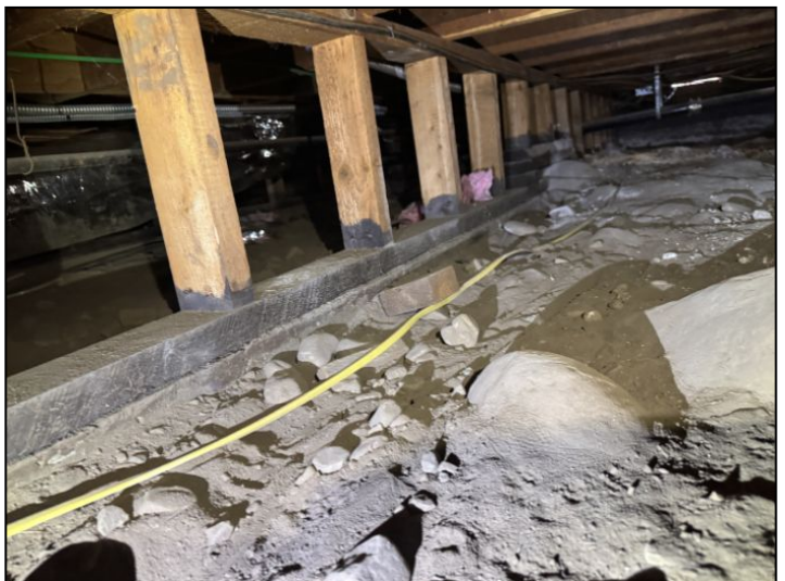
unsupported romex - on ground
