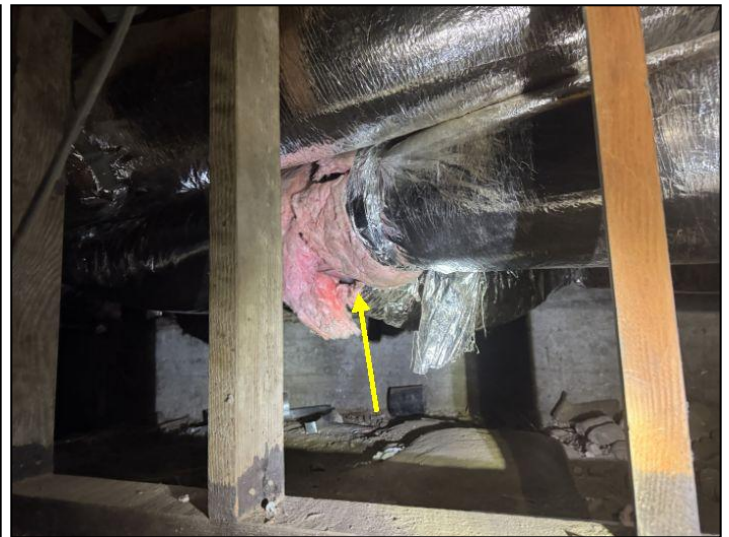
damaged insulation to ducts
