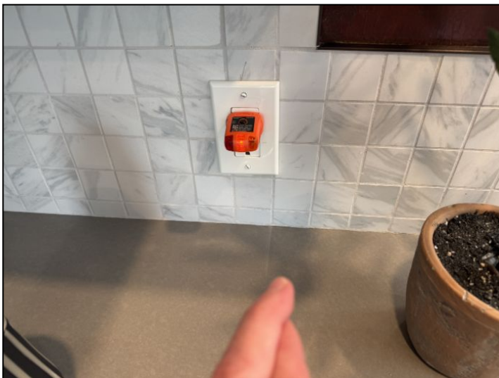
open ground/no gfci
