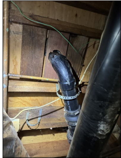
location of active leak
