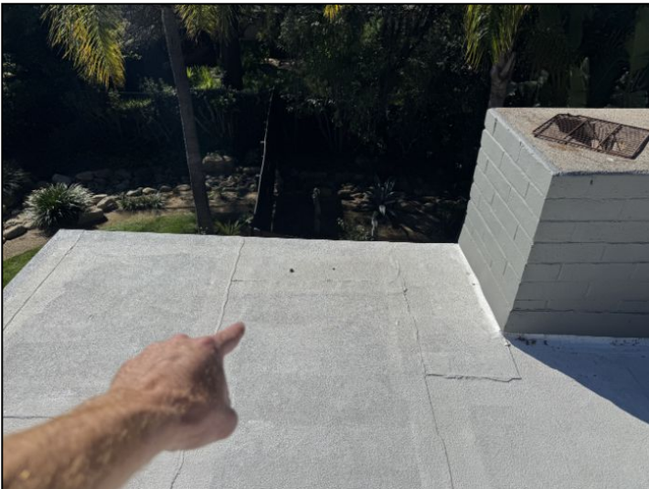
soft spot on roof
