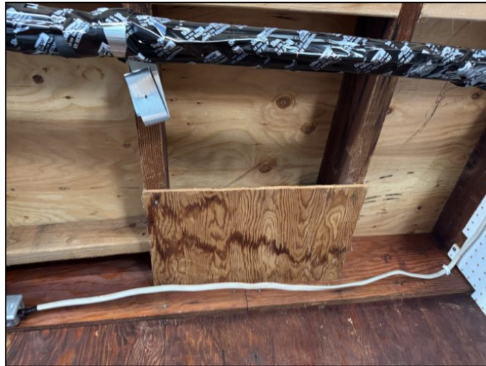
dry moisture staining
