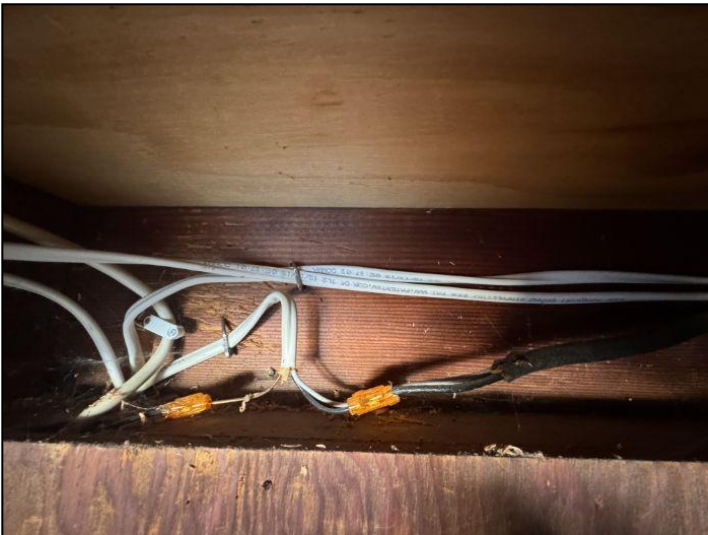
exposed connection in garage
