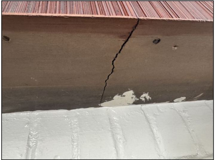
crack in mantel
