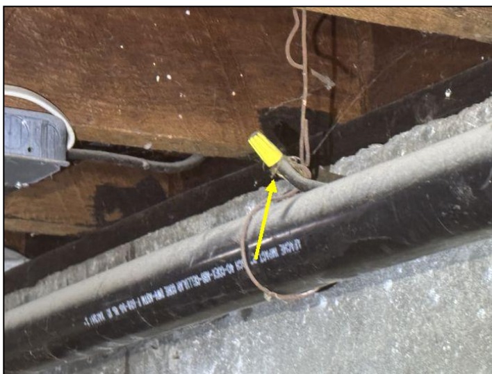
capped cut cloth wire outside junction
