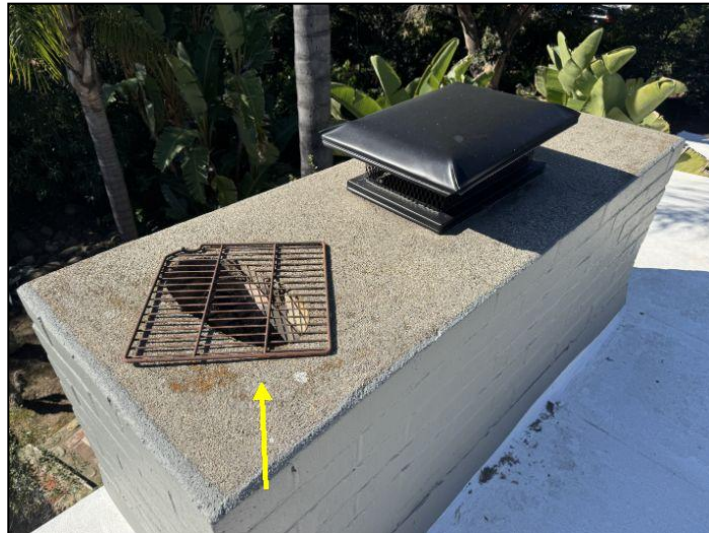
missing spark arrestor and rain shield
