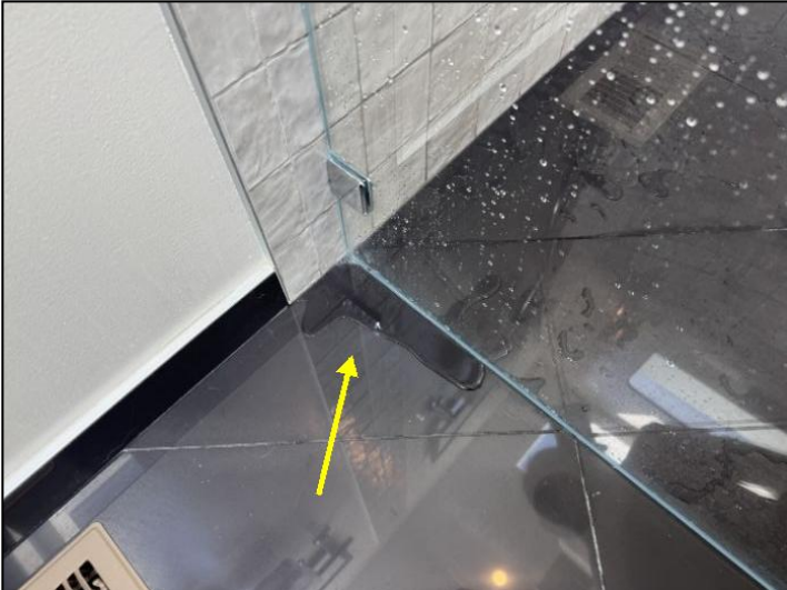
leaking shower wall
