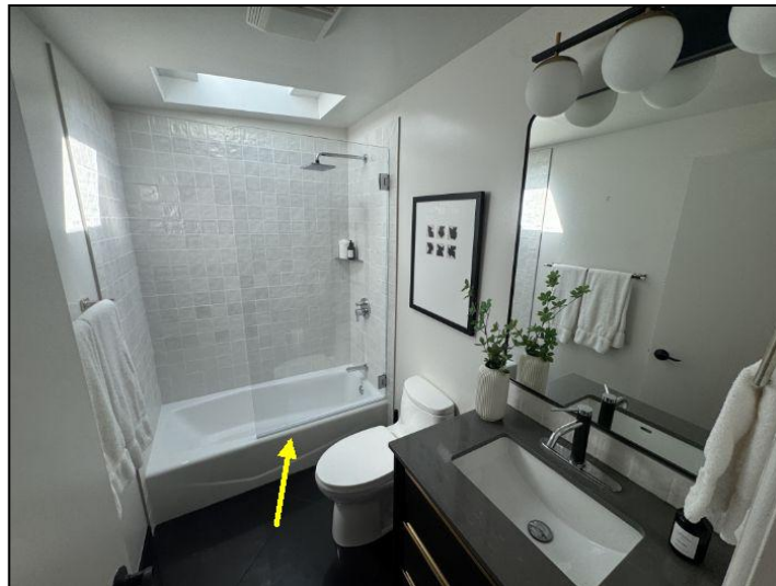
glass panel leaking
