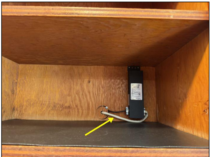
exposed romex in cabinet
