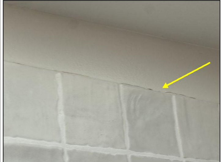
seal gap and cracks- above shower walls
