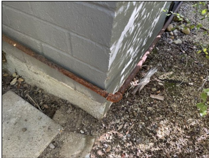
gas line rust
