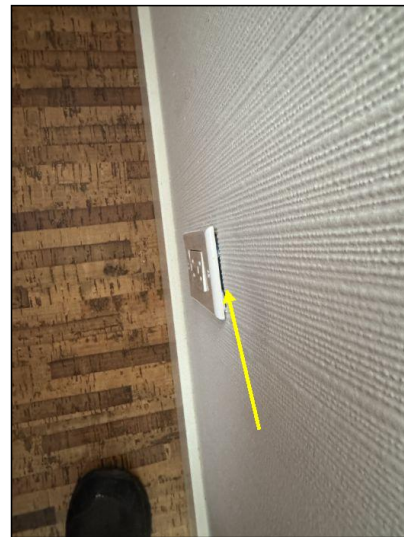
seal gaps around electrical
