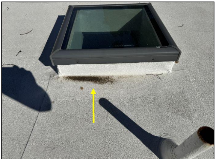
moisture pooling and debris
