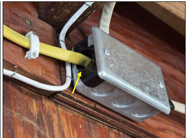
no clamp or bushing - defect
