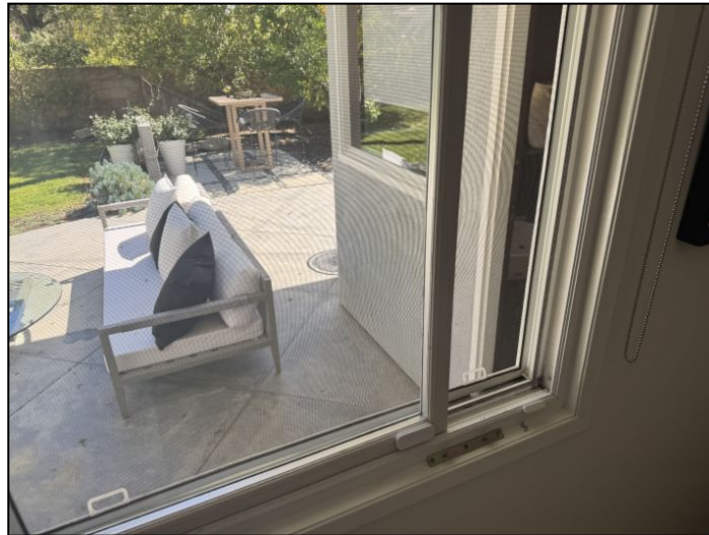
tight window, recommend maintenance
