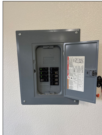
100 amp sub panel
