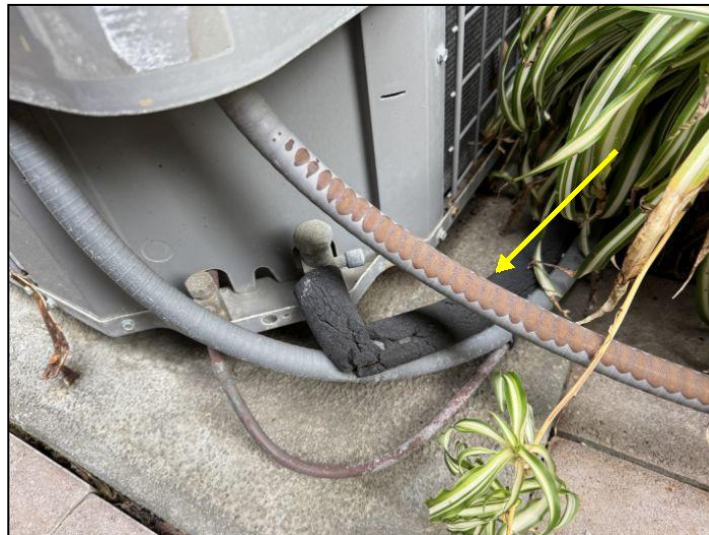
discoloration of conduit - possible exposure
