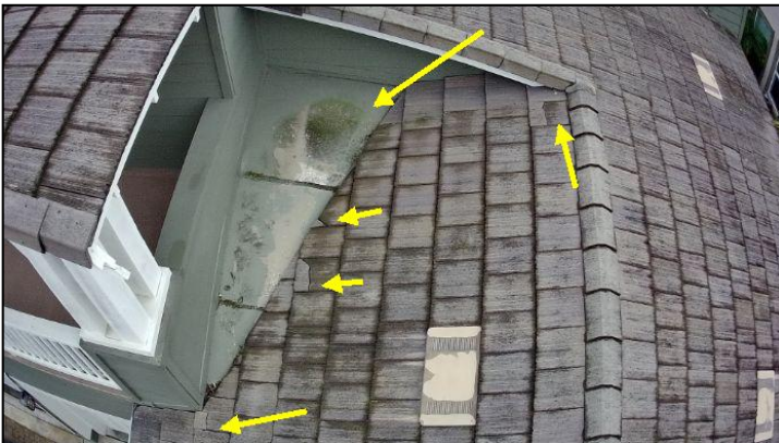
moss build up and cracked tiles
