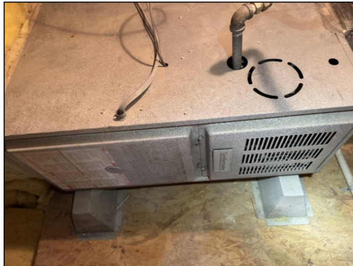
overspray on furnace
