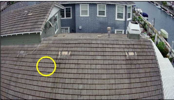
crack in tile
