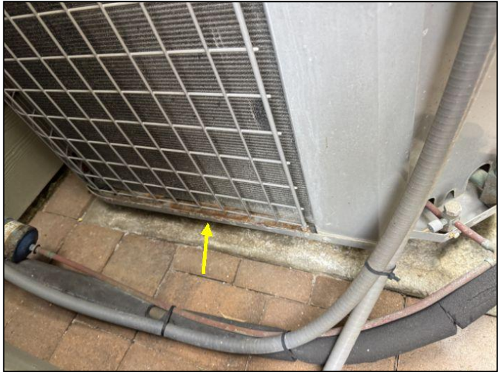
rust in unit
