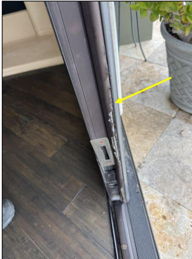
damage to weather stripping
