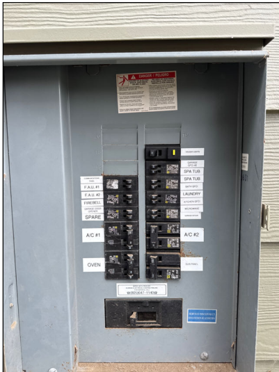
200 amp main panel
