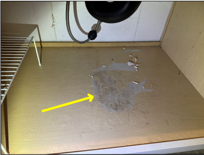
Previous leak - laundry
