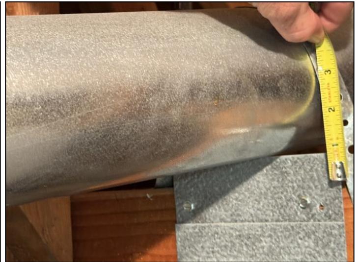
less than inch clearance
