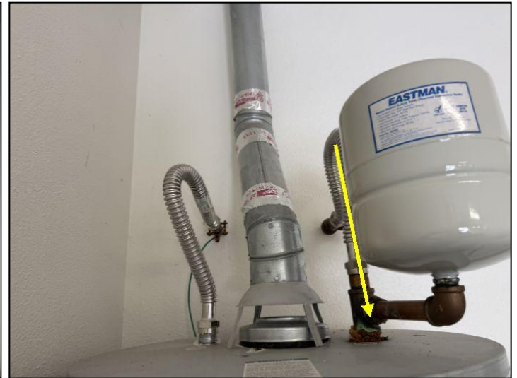
corrosion on water heater plumbing connection point
