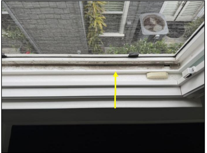
dirt on window sills
