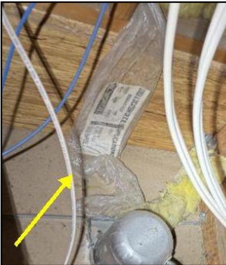
trash in attic - recommend removal
