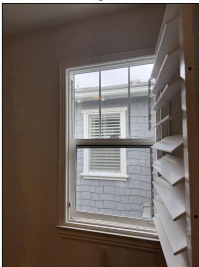
right window top of stairs - broken
