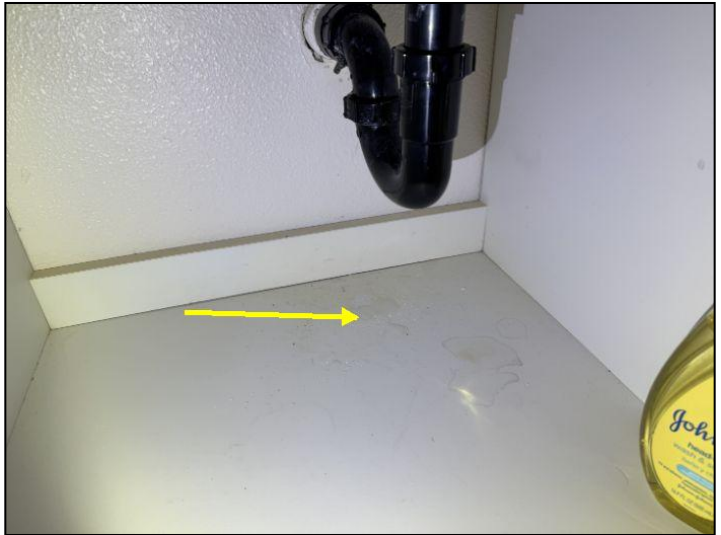
active leak - upstairs left bathroom
