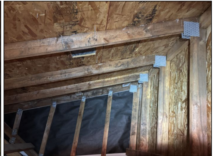
staining on trusses
