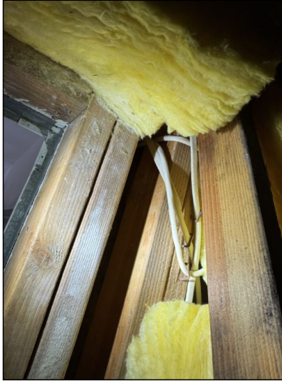
conductors next to access
