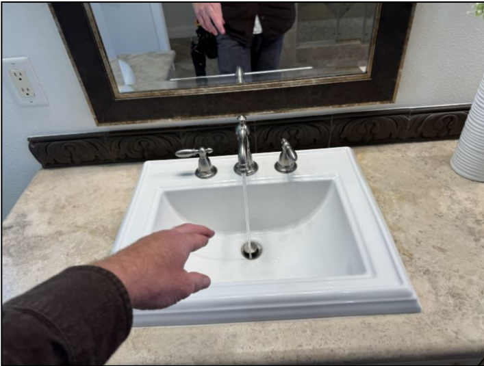
slow flow on left sink in master
