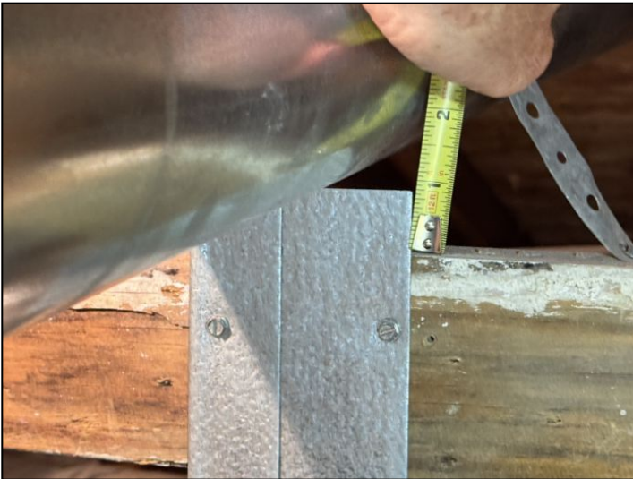
less than inch clearance
