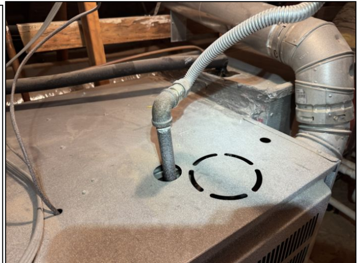
missing sediment trap(s)
