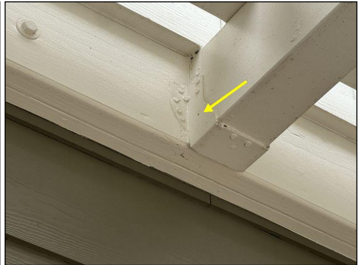
missing fastener on patio
