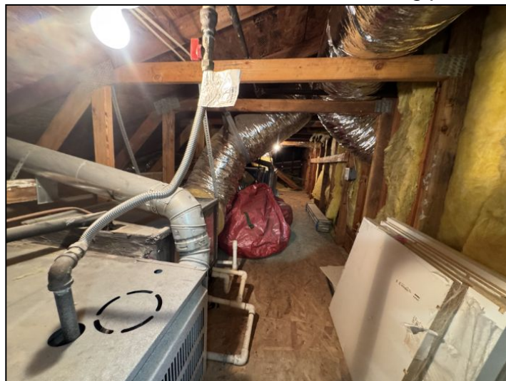
access to furnaces - photo for client
