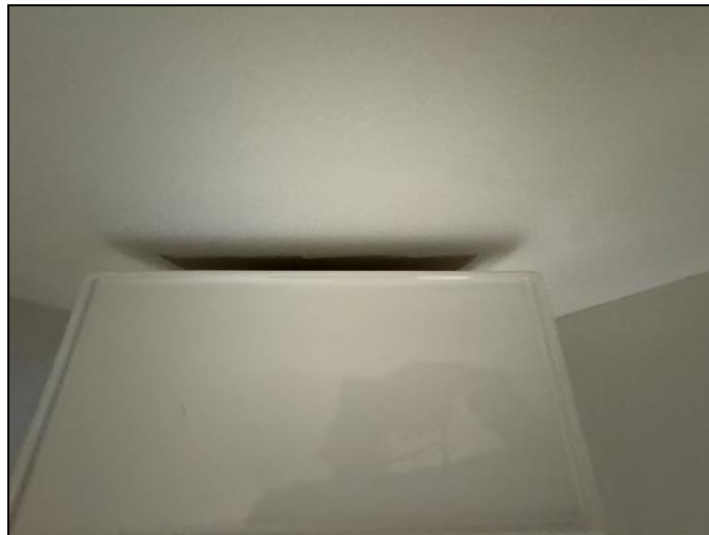
no paint behind toilet - master
