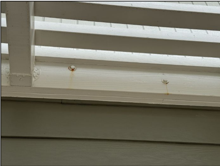
rust on bolts
