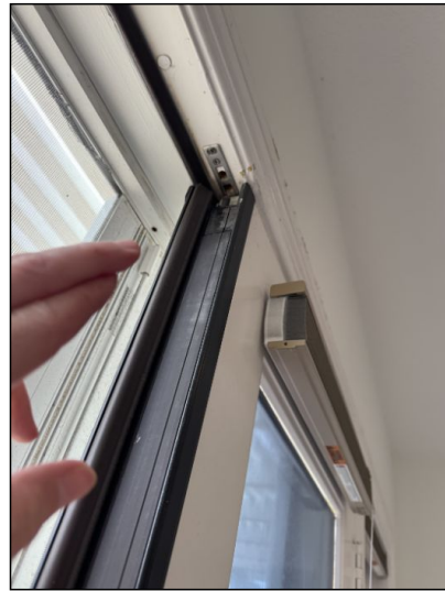
difficult lock patio door bedroom
