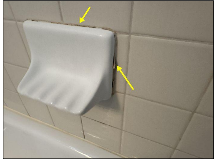
bathroom 3 - missing caulking
