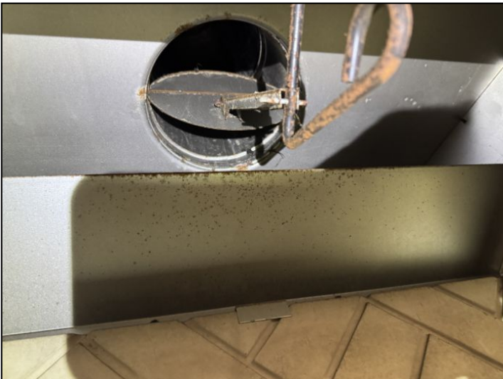
Patio room - slight rust - no damper clamp
