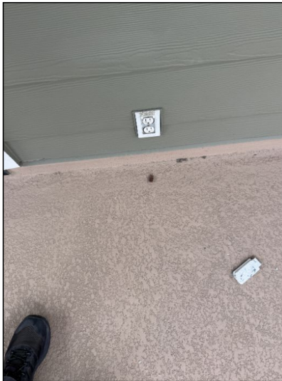
non functinal GFCI and broken cover - patio
