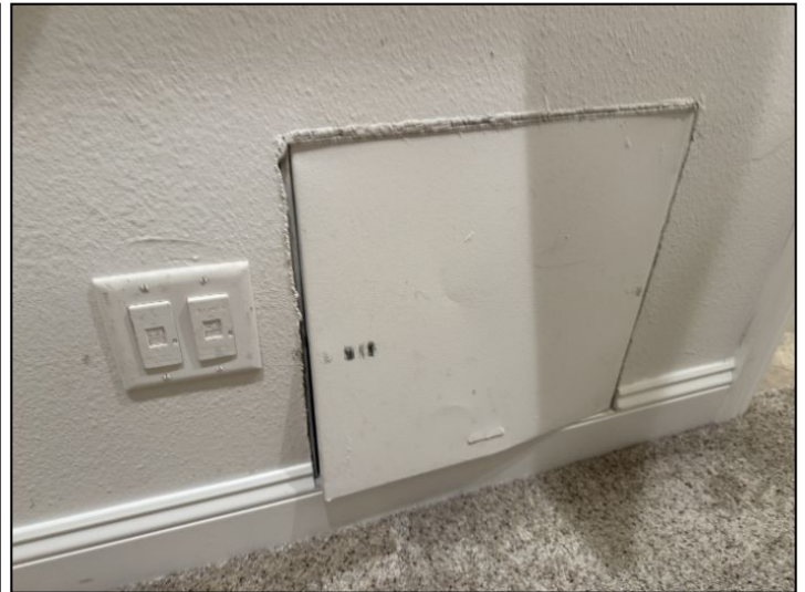
access stuck open
