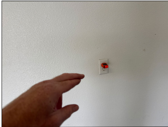
Missing gfci protection
