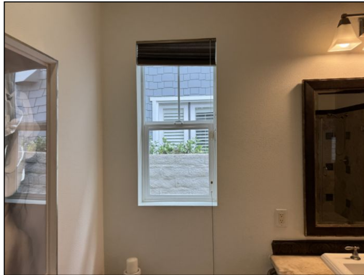
missing screen bathroom window
