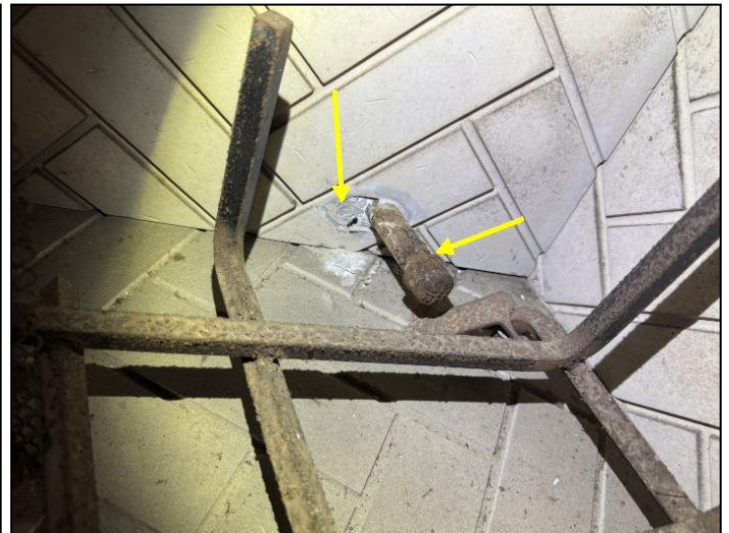
scaling rust on capped gas line. damage to connection point.
