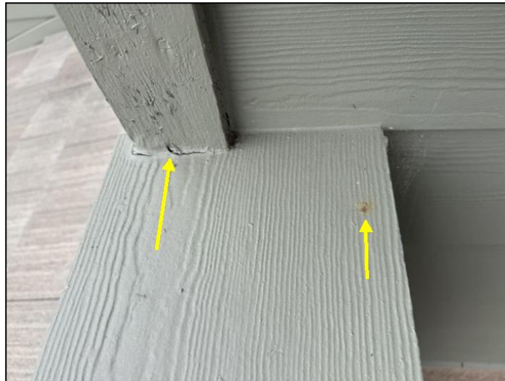
crack and rusted attachment
