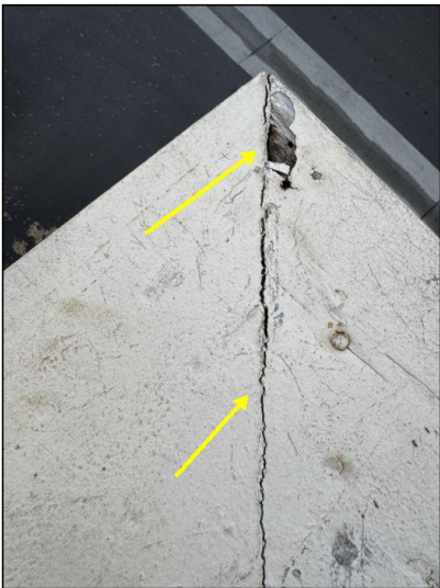
damage to exterior-patio
