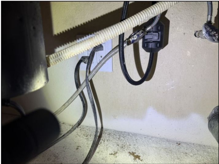
recommend GFCI under sink
