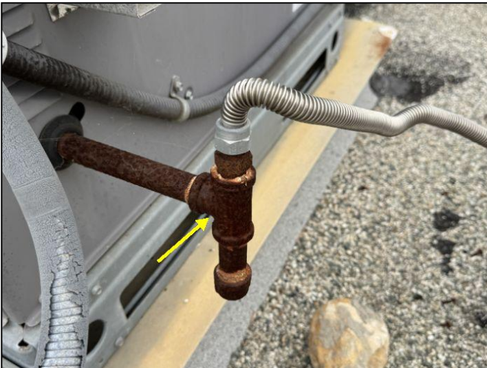
rust on gas line
