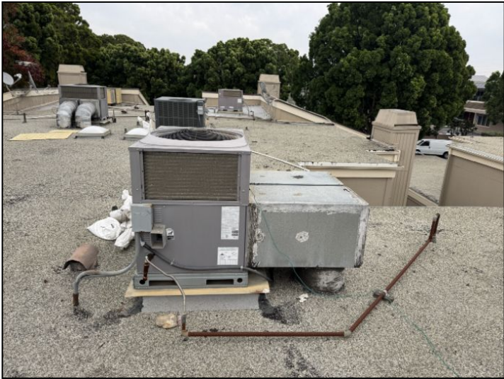
recommend review of unit as a whole by qualified contractor
