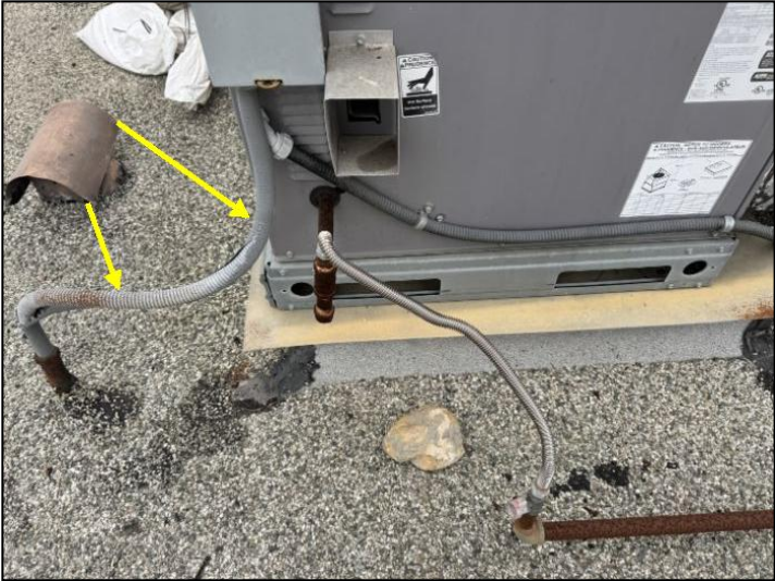
damage to electrical conduit
