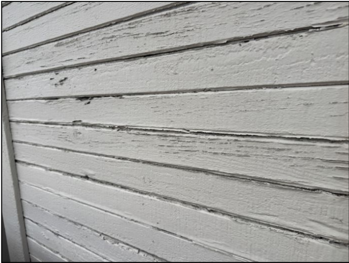
exterior chimney wood damage
