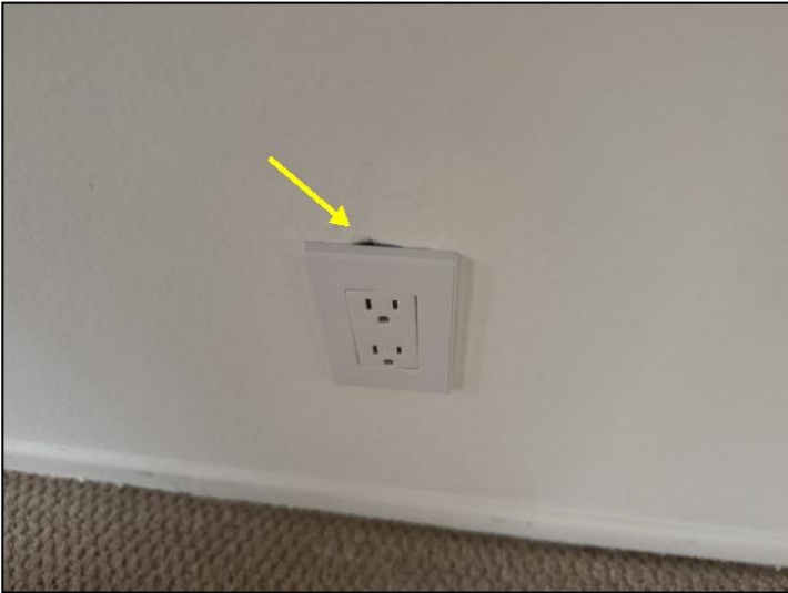
Bedroom-gap around outlet
