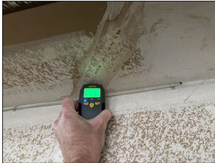
moisture staining in garage- low moisture at the time of the inspection.
