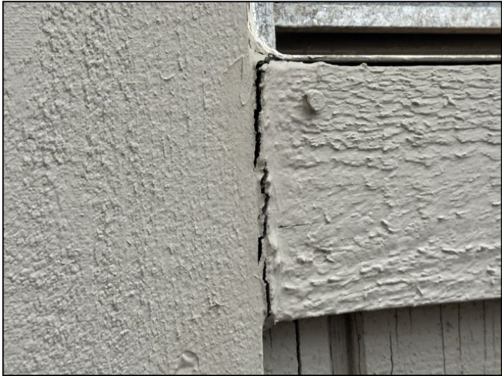
seal all gaps and cracks
