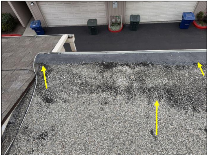
excessive sealant and missing gravel on roof
