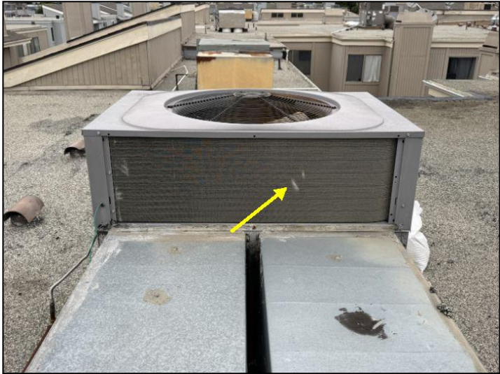
damage to fin observed
