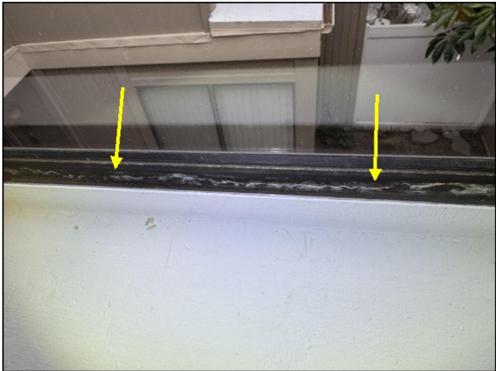
signs of moisture
