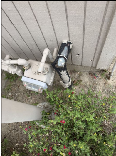
damage to insulation on exterior water line
