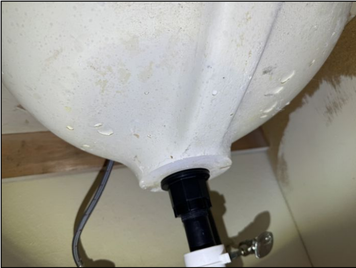
functional but cracking underside
