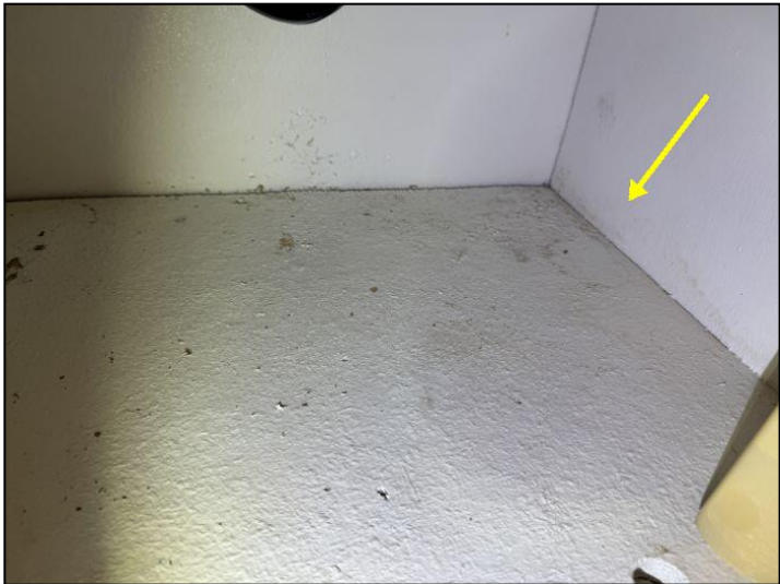
previous moisture staining
