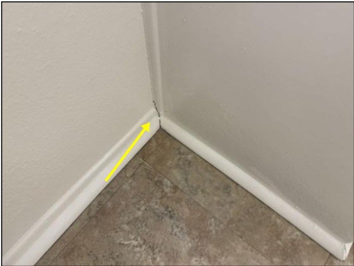
seal crack, half bath wall
