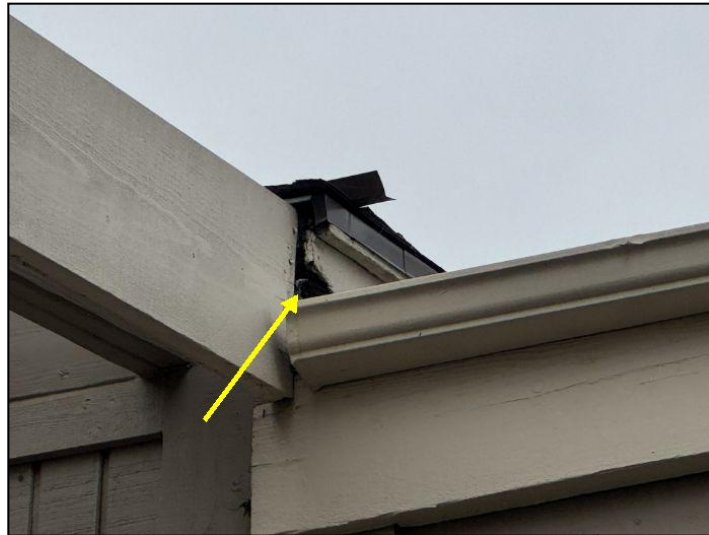
rot/wood damage above patio
