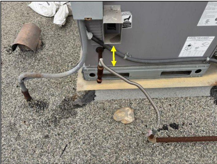
hot exhaust directly onto flex gas line
