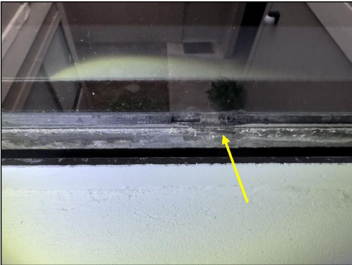
efflorescence and deterioration of seal
