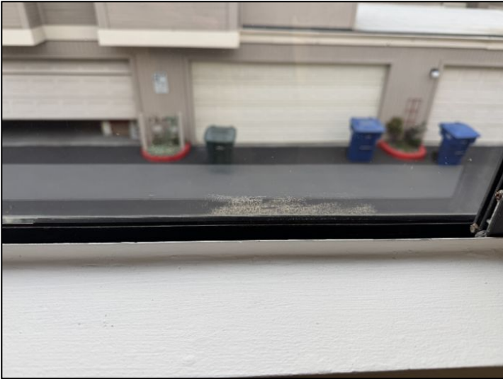
overspray on windows
