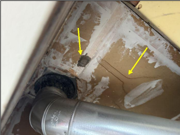
moisture staining/pest nest
