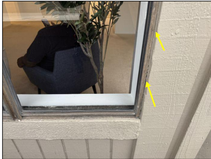
seal around windows
