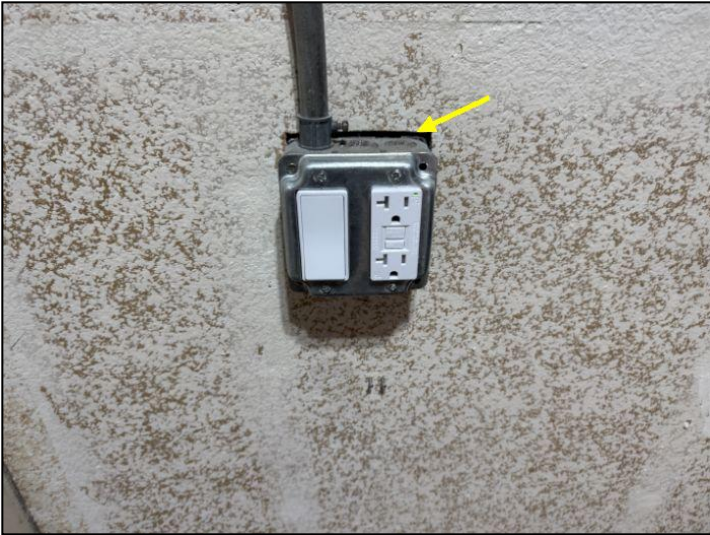
gap in firewall
