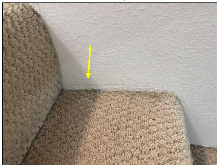
marks from carpet installation
