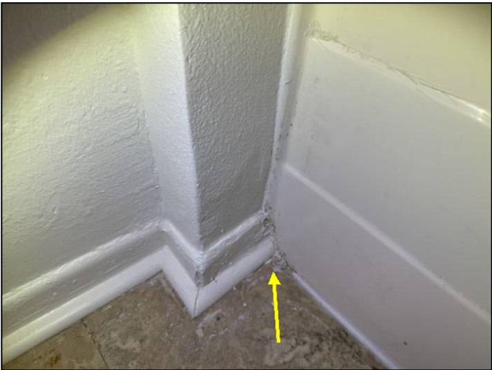
painted over damage
