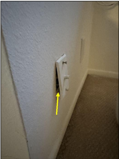
loose outlet cover - fireplace room
