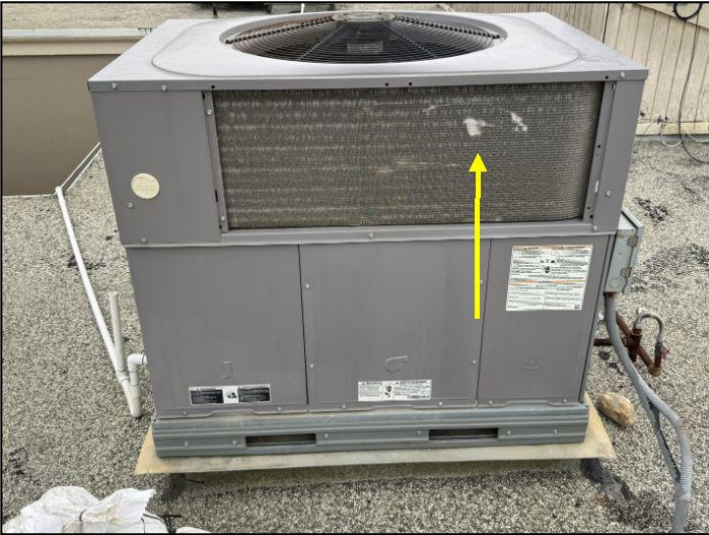
damage to fins
