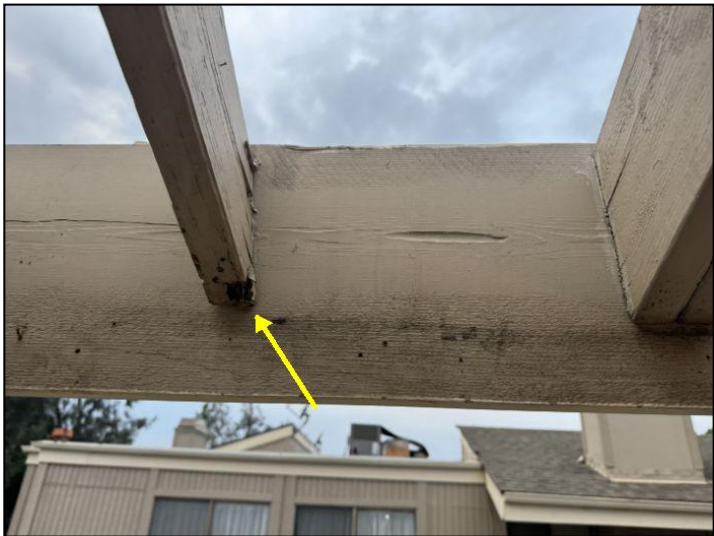
possible pest damage
