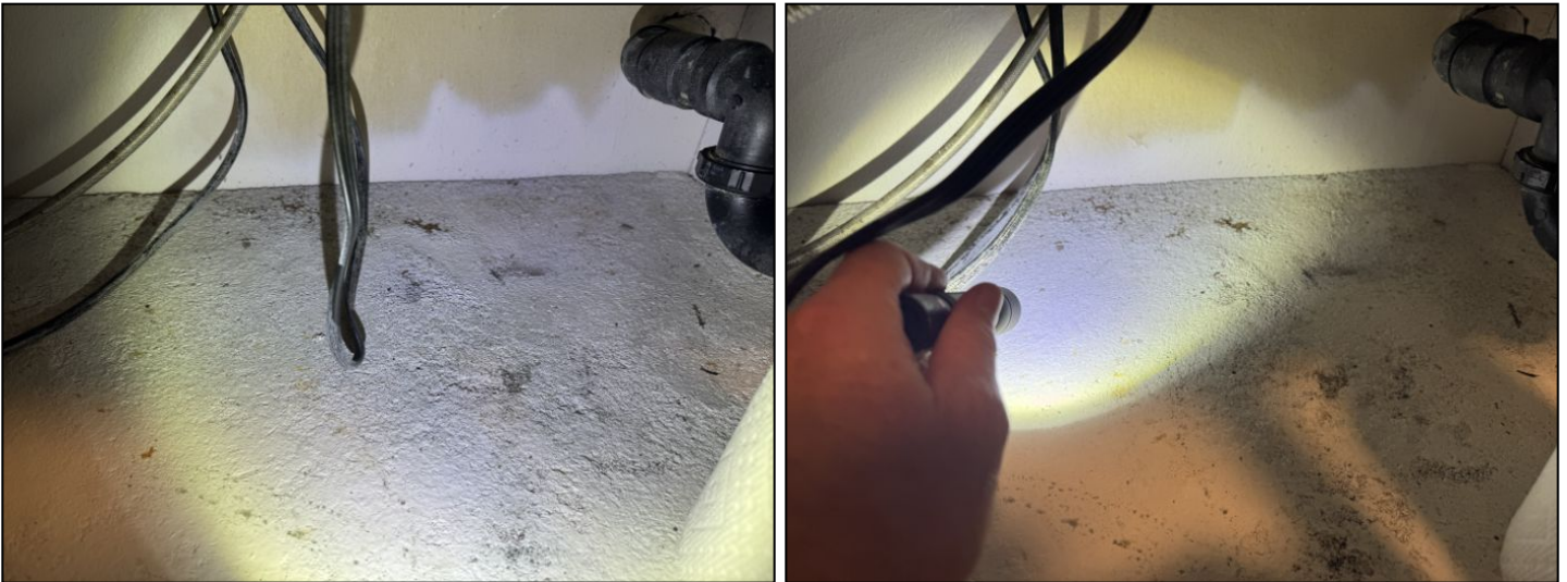
aged under sink/past moisture/possible microbial growth
