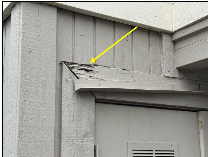
possible wood destroying insects/moisture damage
