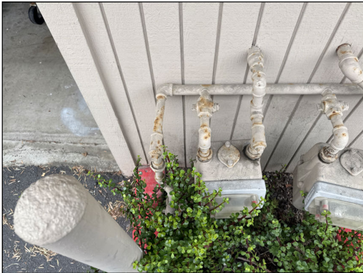
main gas valve
