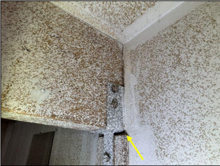
gaps in walls
