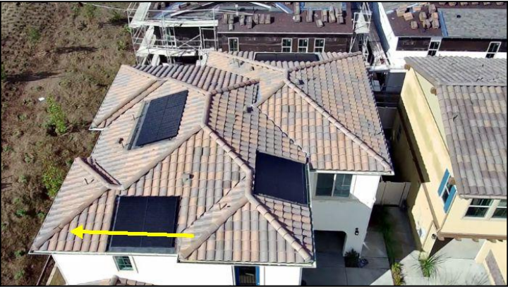
possible cracked tile
