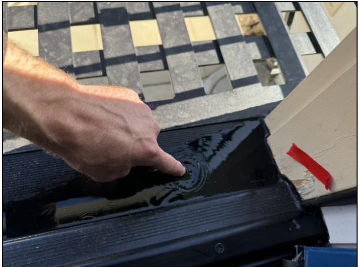
improper fall/moisture settlement
