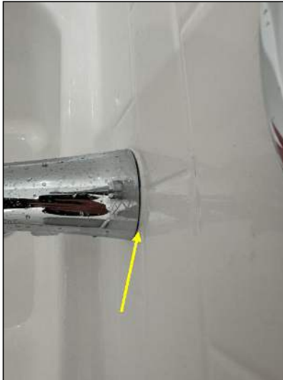
gap at shower faucet-upstairs hallway
