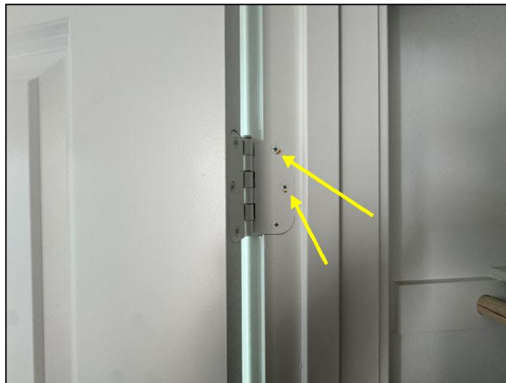
rusting screws-closet next to front door
