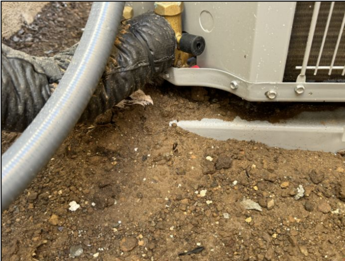
mud flow under exterior unit
