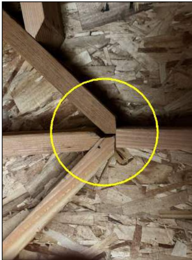
separation of attic framing
