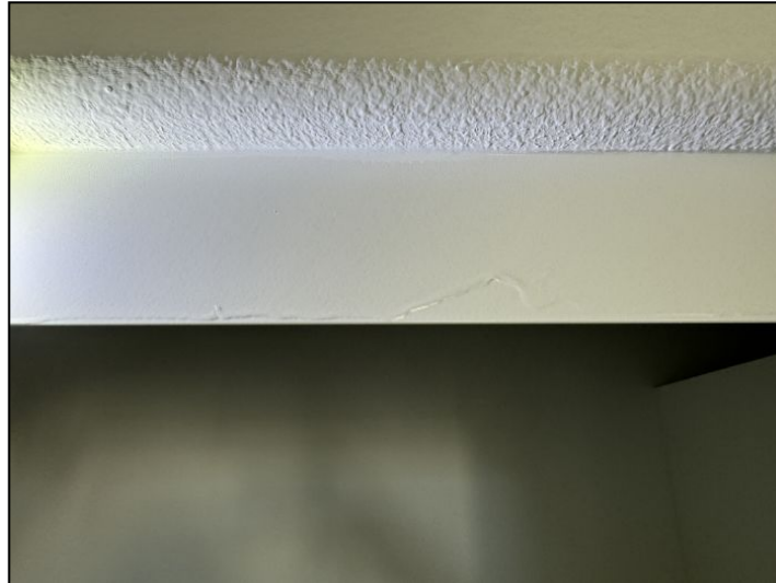
dripping paint above closet
