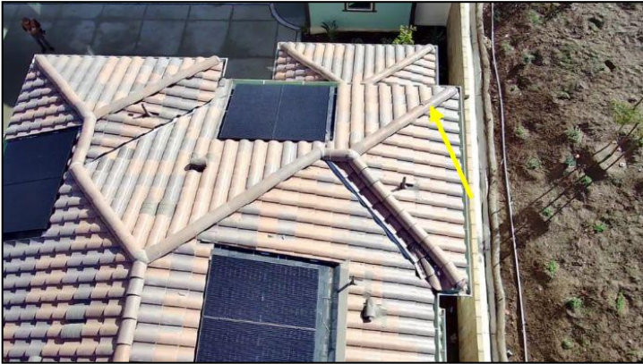
possible cracked tile
