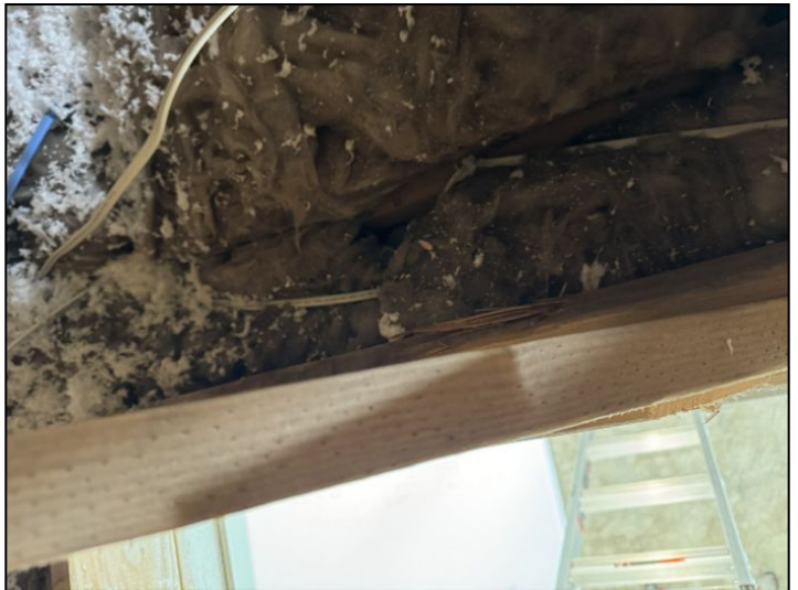
electrical conductors right next to access
