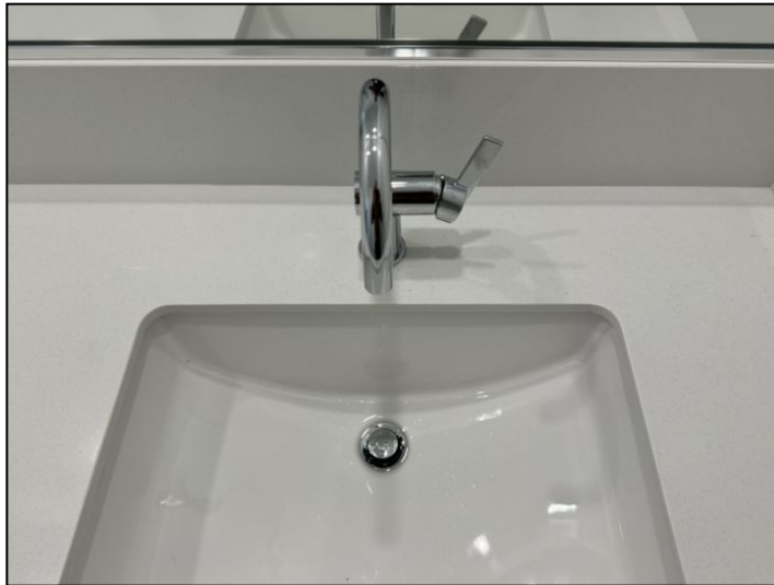
no hot water - hallway bathroom
