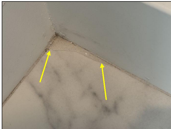
excess grout/cracking -master toilet
