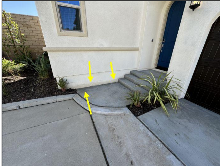
signs of moisture
